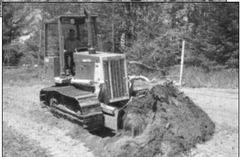
Norm Pestka uses a Komatsu D38E-1 dozer to smooth a ditch on a job near U.S. Highway 64 west of Ontonagon, Michigan.
